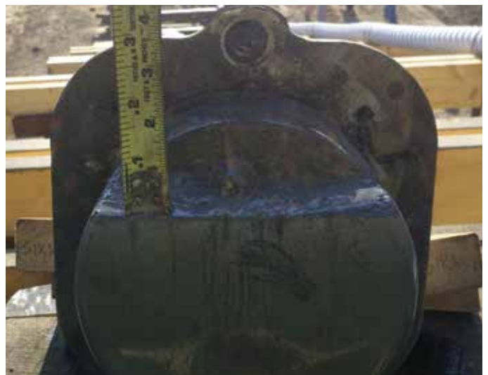
Grout 2 outlet end cap has void and soft grout.
