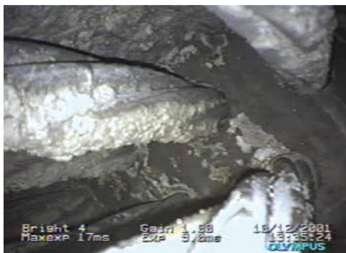
Fig. 3—Typical voids adjacent to anchor plates in draped tendons.
