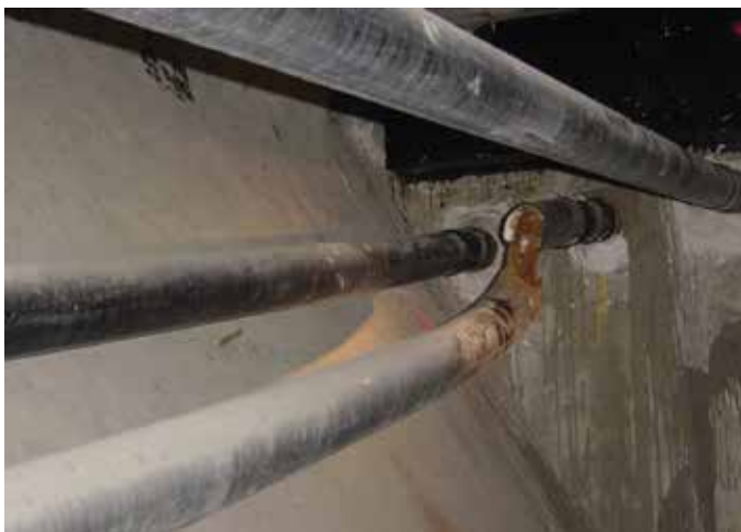
Fig. 2—Failed draped tendon found during inspection on May 22, 2007.
