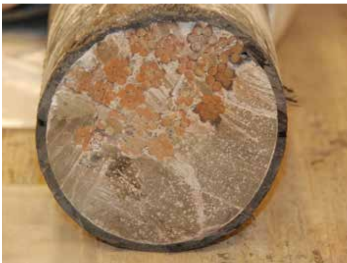
Fig. 6—Typical grouted draped tendon, indicating it is not possible to surround strands with grout.
