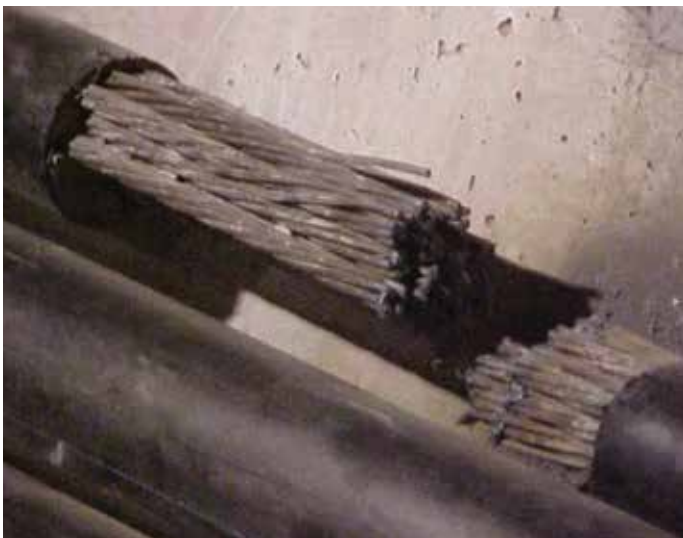
Fig. 9—Tendon T1 with completely cut strands.
