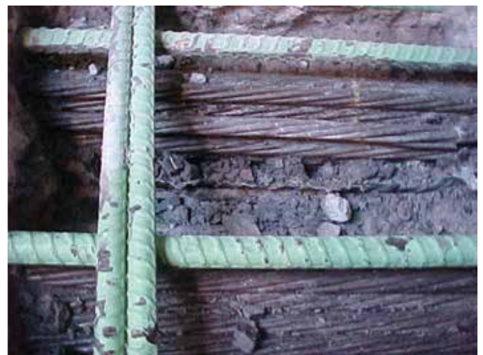
Fig. 8—Close-up of exposed strands in portion of tendon embedded in bottom slab.
