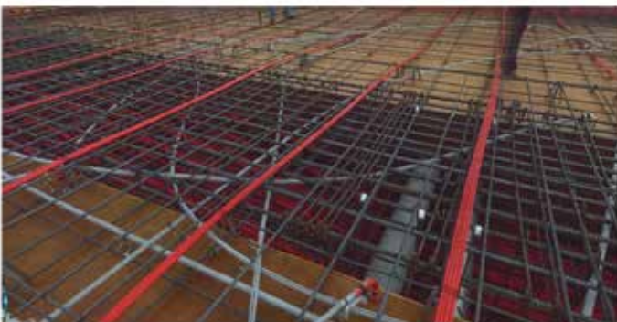
Fig. 2—Extracted digital image of a post-tensioned slab from a laser scan. (Photo courtesy of Hensel Phelps Construction)
