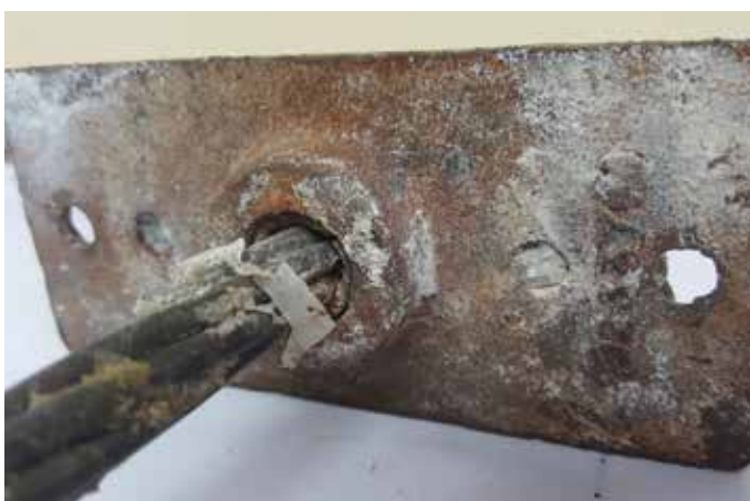
Fig. 15—Specimen No. 3: anchor, bearing side.
