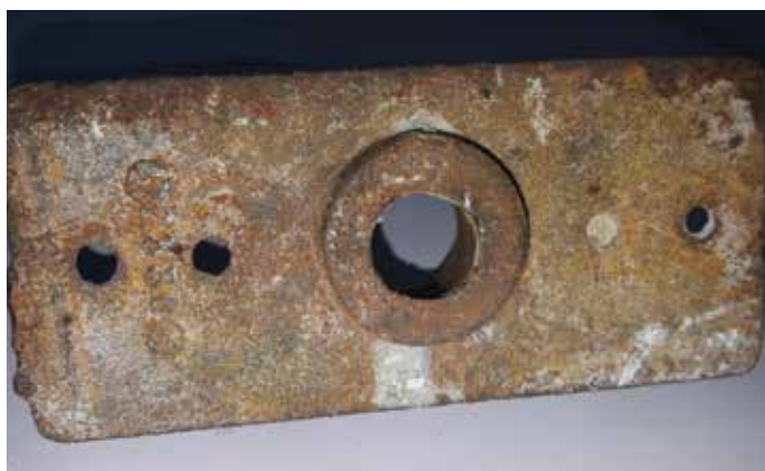
Fig. 10—Specimen No. 2: anchor, bearing side.
