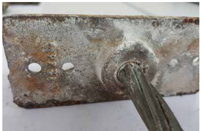
Fig. 21—Specimen No. 6: anchor, bearing side.
