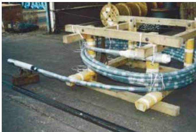
Fig. 2—Post-tensioning 40 mm (1.57 in.) diameter CFCC with pre-installed anchoring devices on both ends.
