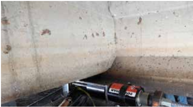
Post-tensioning cable with load cell
