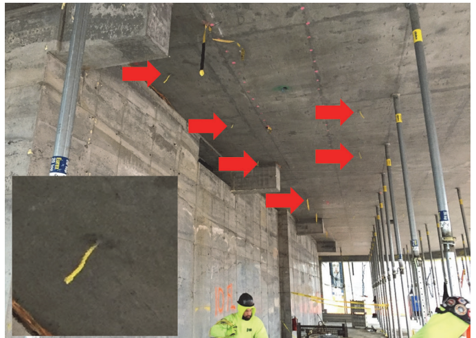
Fig. 5—Nylon ropes showing underneath slab.
