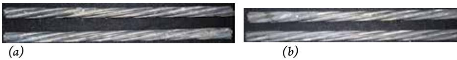
Fig. 13—Corroded strands near Port C of: (a) control ISG specimen; and (b) control TSG specimen.
