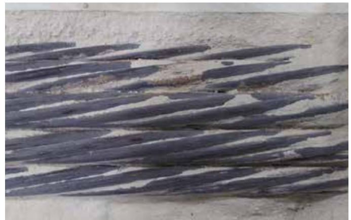
Fig. 9—In-place corroded strands near Port C drying TSG specimen.
