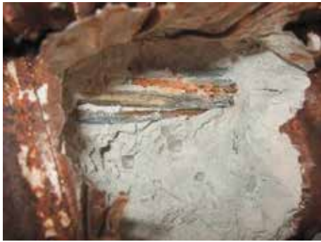
Fig. 1—Deficient grout in PT tendon in Sicily, Italy (Anania et al. 2018).
